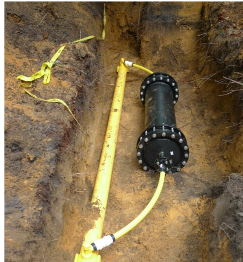
Figure 15. Test rig under G-gas conditions.
