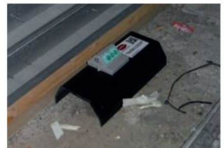
Fig 2: GT sensor mounted on upturned gutter
